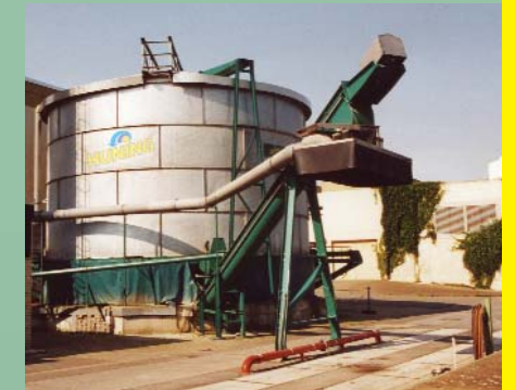
Sewage sludge silo 450 m 3 with loading conveyor and aspiration system
