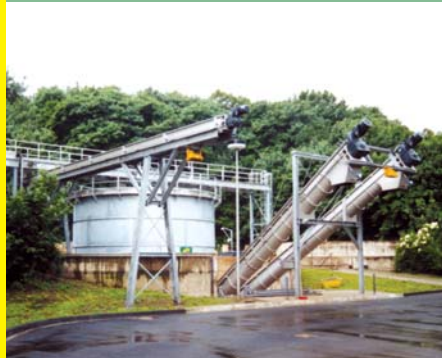
Sewage sludge silo 380 m 3 discharge and loading screw in tandem design
